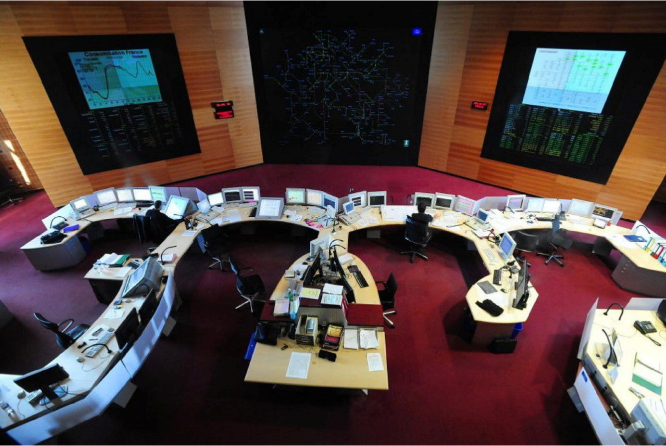
Rte Control room
